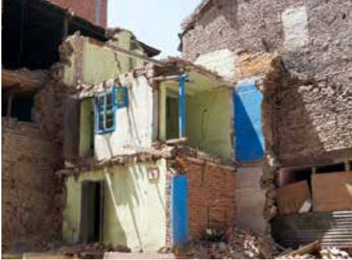
Raghuchour village, after the earthquake
