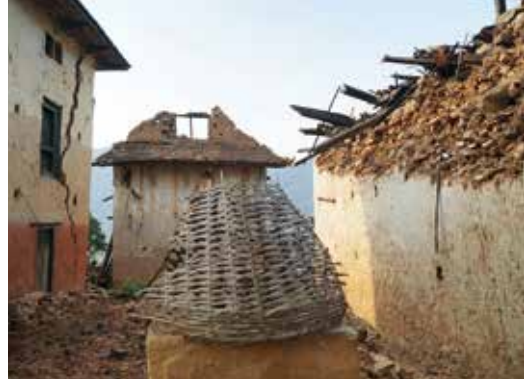
Raghuchour village, after the earthquake
