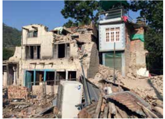
Raghuchour village, after the earthquake
